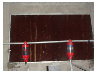
Cooling Pads for cooling of air in the shed.
