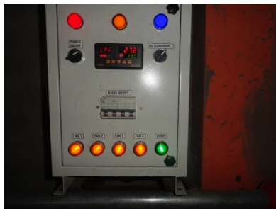
Automatic Temperature control unit.
