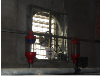
Exhaust fans for exchange of air inside the shed.
