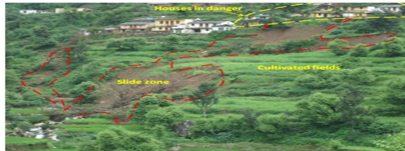
Fig. 6. Land unsuitable for development (slide zone) has built up and cultivation, Uttarakhand. Picture taken before the disaster. Source: Geological Survey of India.
